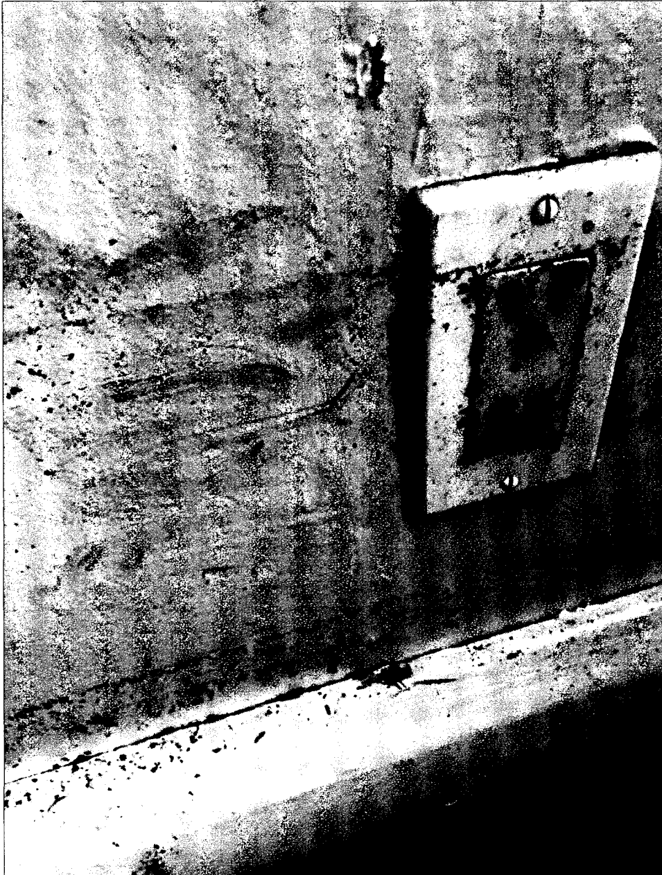
Figure 9: View of electrical socket plugged with debris
